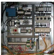
Complex electric controls are thoroughly reviewed.
